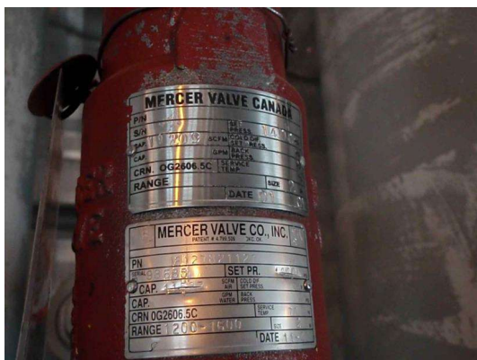
PSV nameplate General Overview
