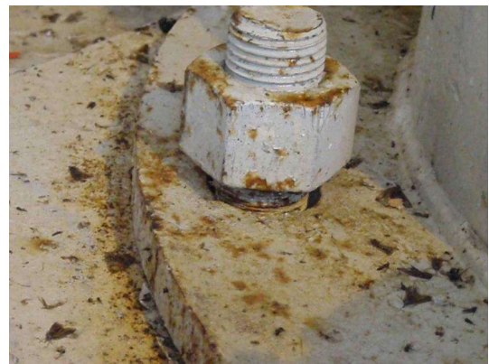
Support Bolt not fastened.
