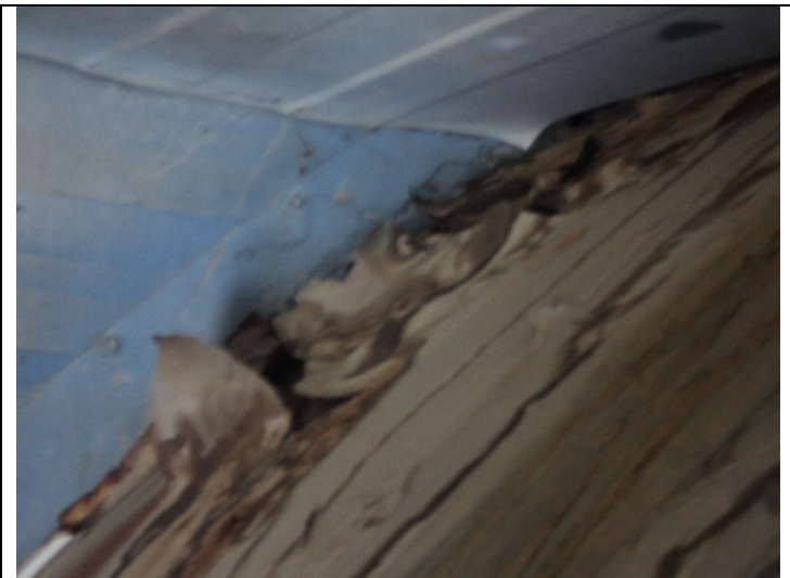
Paint peeling at 12 O'clock
