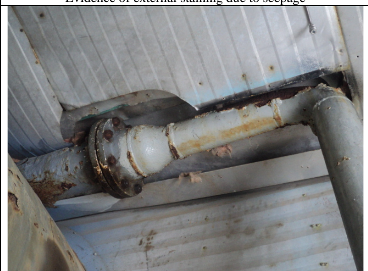
General Overview of Inlet piping
