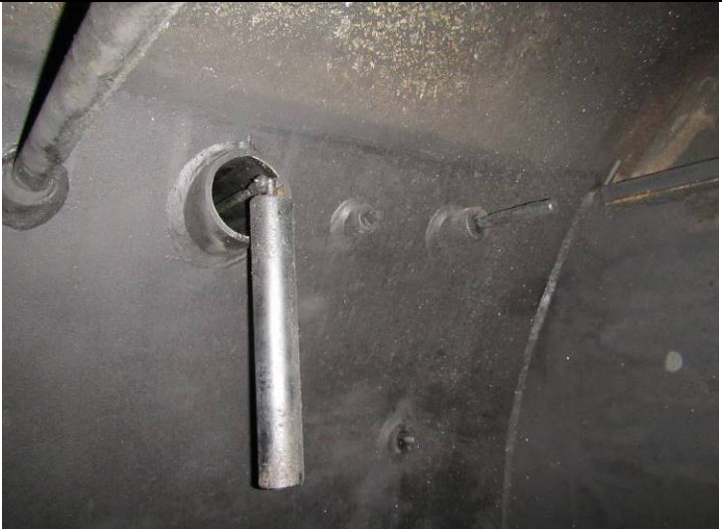
High-level float and thermowell
