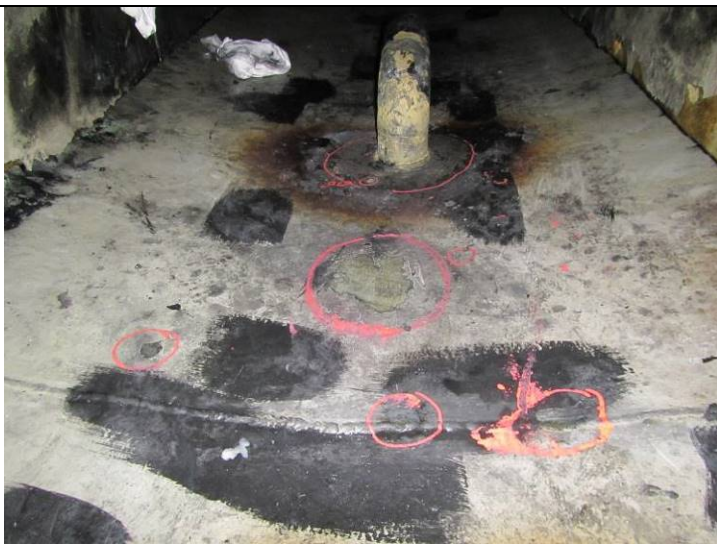
Overview of coating damage in back-end
