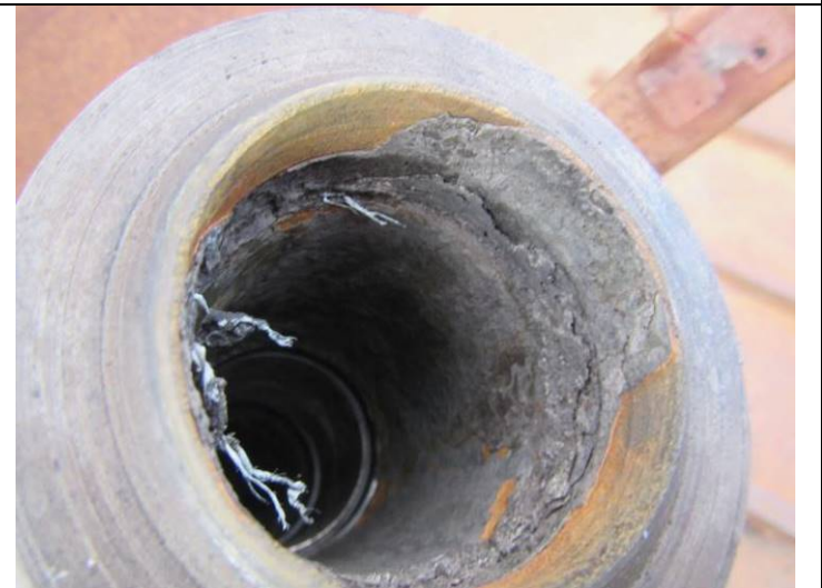
Corrosion on 2 inch threaded piping off gas boot
