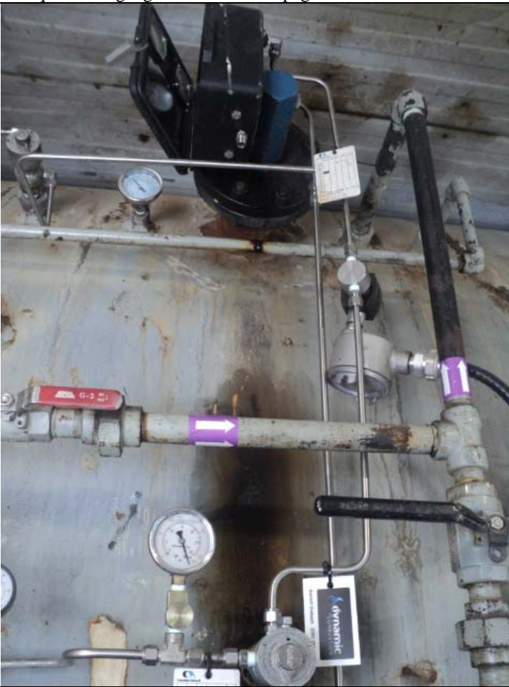
Evidence of external staining due to seepage
