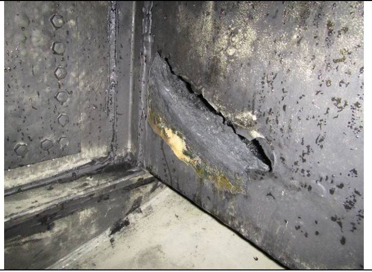
Back-end diffuser is corroded out
