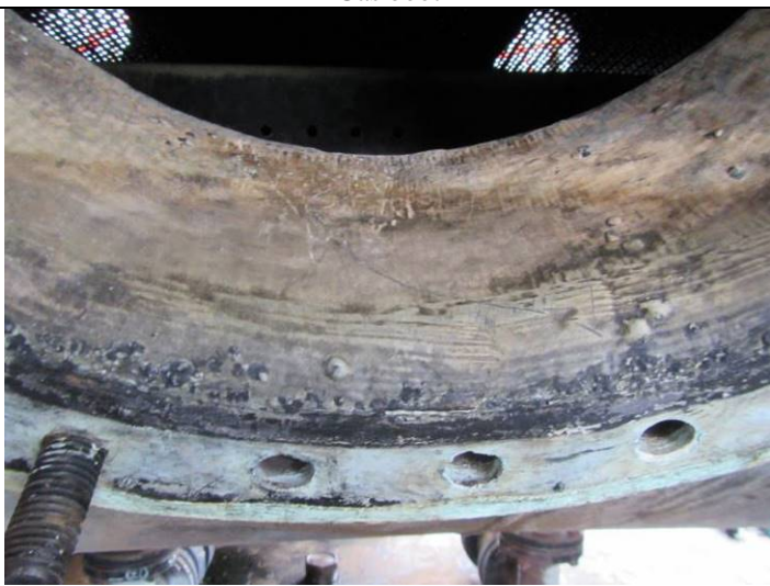
Small diameter coating blisters on manway
