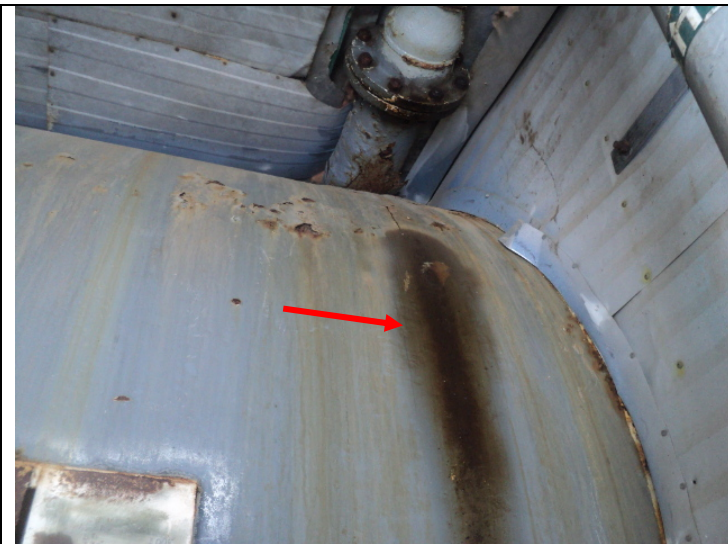
Evidence of external staining due to seepage
