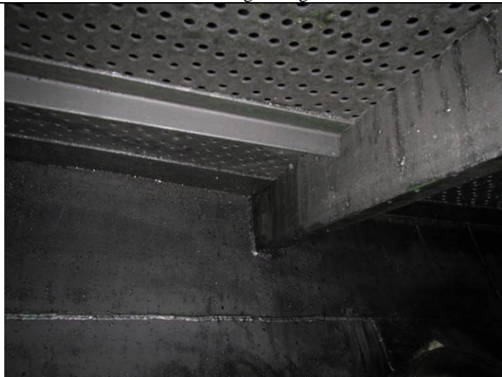
Screens supports are in good condition – no corrosion or mechanical damage noted
