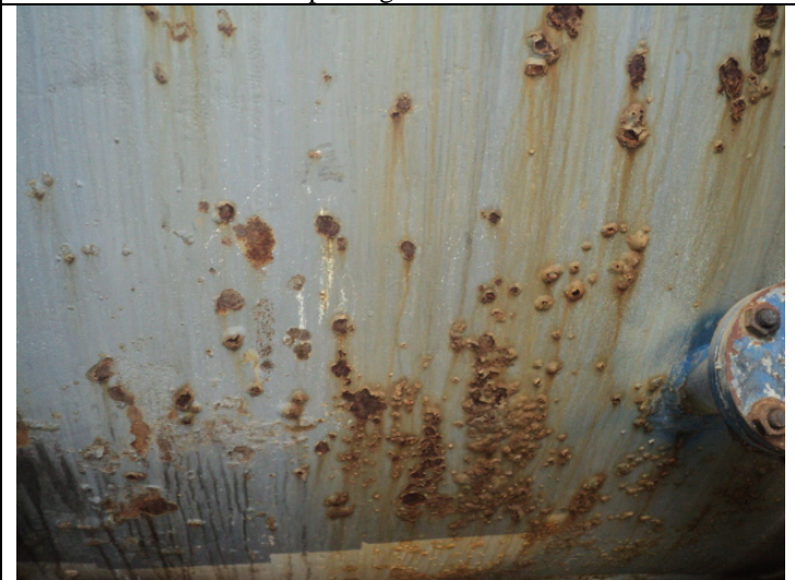
Spotting external corrosion on shell
