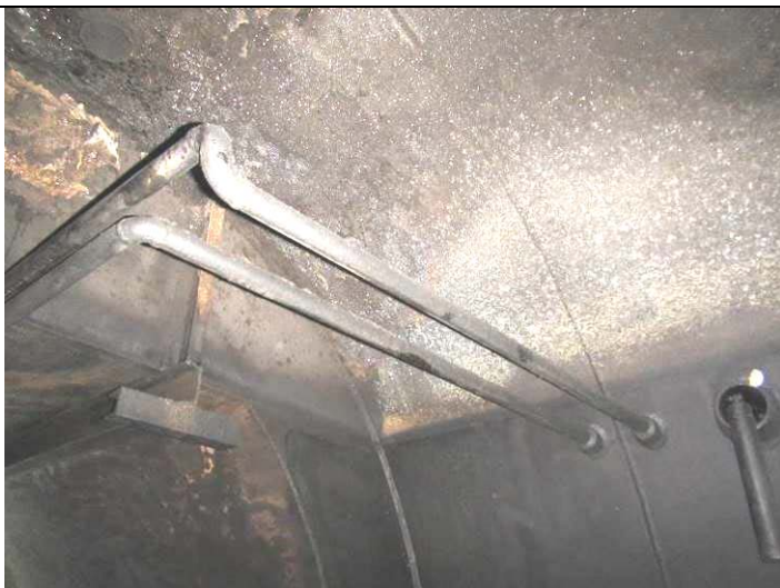
Fuel gas pre-heat piping
