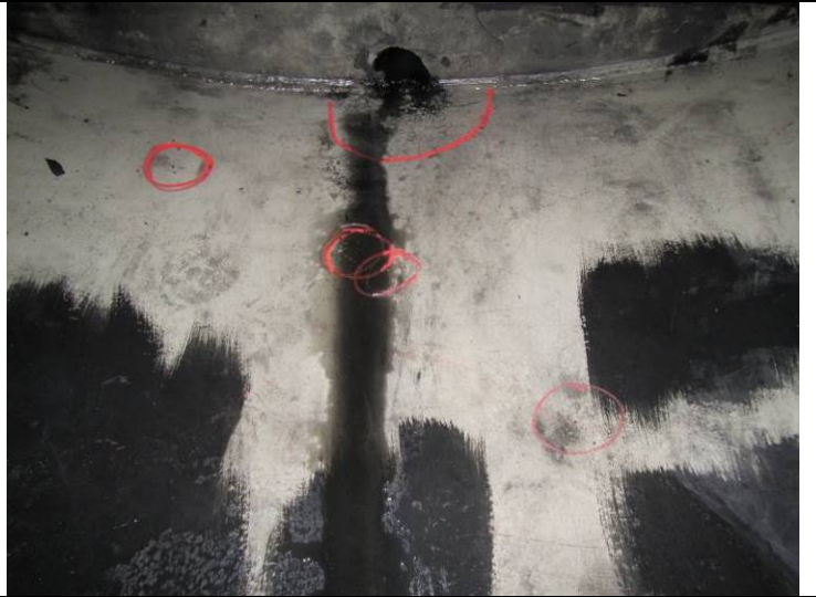
Coating damage at the north side of the back-end
