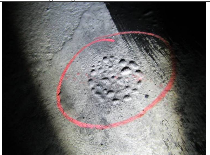
Small diameter blistering on bottom shell
