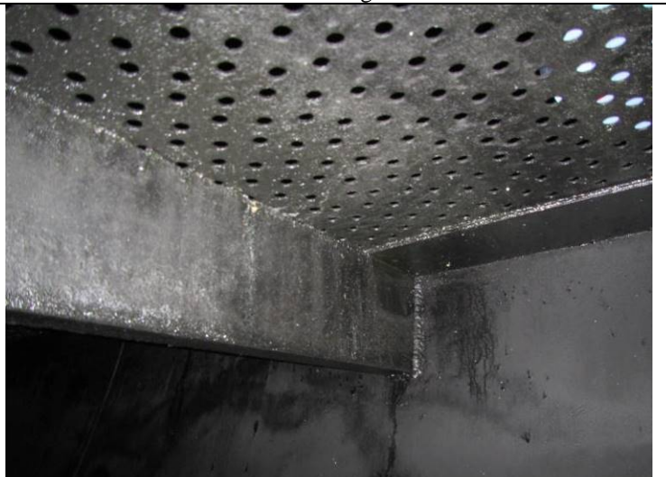
Screens supports are in good condition – no corrosion or mechanical damage noted
